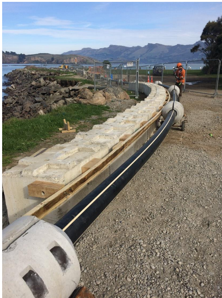
Photograph 2: Governor Bay Submarine Pipeline String
