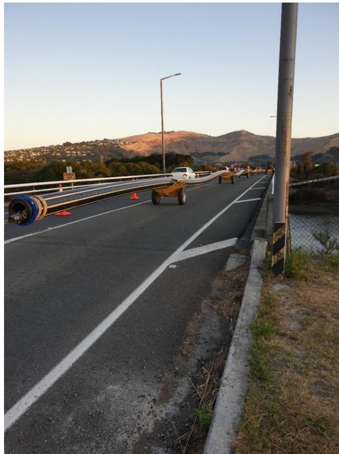
Photograph 3: DN355 PE100 pipe string being positioned prior to the horizontal directional drill under the Heathcote River
