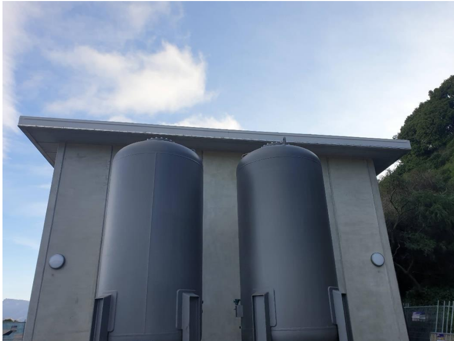
Photograph 5: Surge Vessels at the SIMEON QUAY PUMP STATION Site
