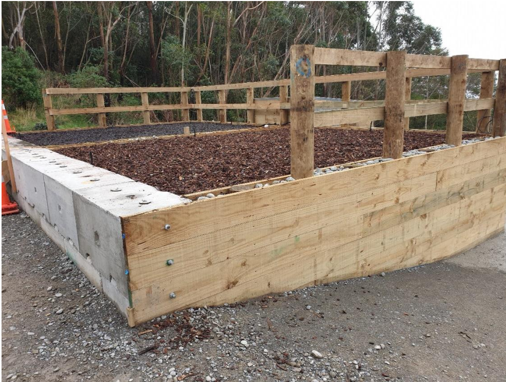
Photograph 7: Biofilter Constructed above tunnel pressure outlet, for odour treatment at the discharge end of the tunnel pipeline
