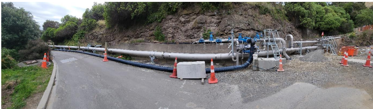
Photograph 9: DN400 SS316 above ground pipeline that was design and constructed to avoid the existing 66 kV buried power cable
