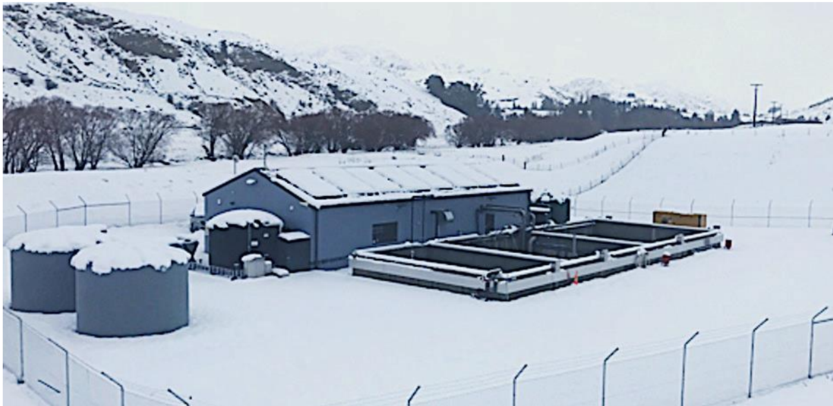
Figure 12 Cardrona wastewater treatment plant (including solar panels) buried in snow - July 2022
