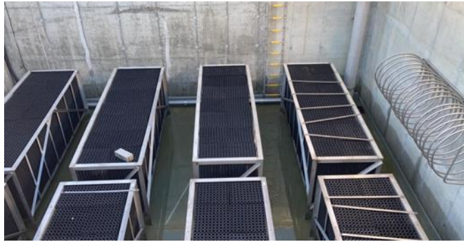
Figure 7 Bioblock installed in the bottom of the SBR tanks. In-tank heating coil shown to the right
