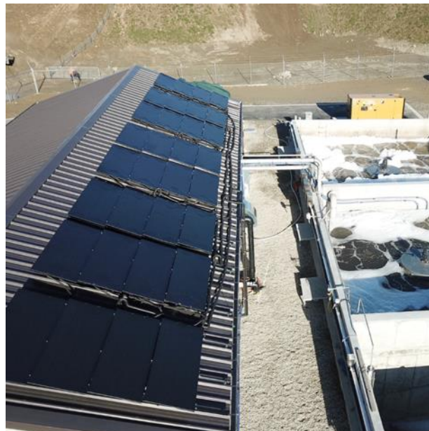
Figure 9 Solar thermodynamic panels on the roof of the treatment plant building
