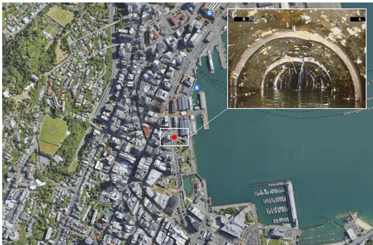
Figure 1: Location of the void and view from within the damaged 450mm EW pipe
