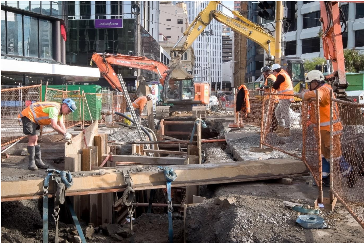
Photograph 2: Trenching works during the four-day shutdown (Credit: Mark Tantrum Photography, Mark Tantrum)
