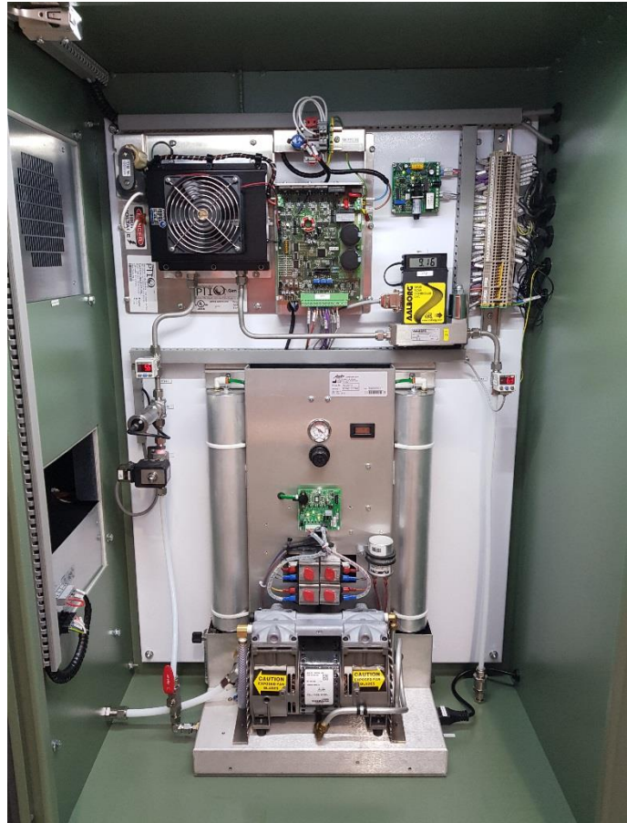
Photograph 8: Major internal components
