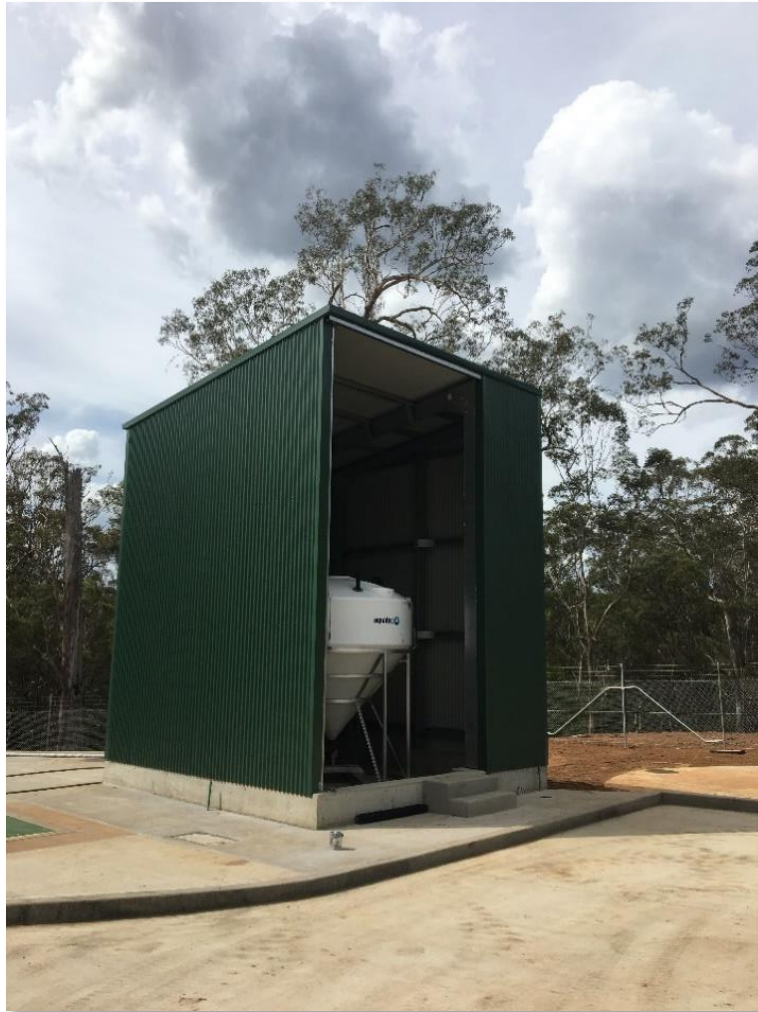
Photograph 4: Example of typical MHL dosing unit
