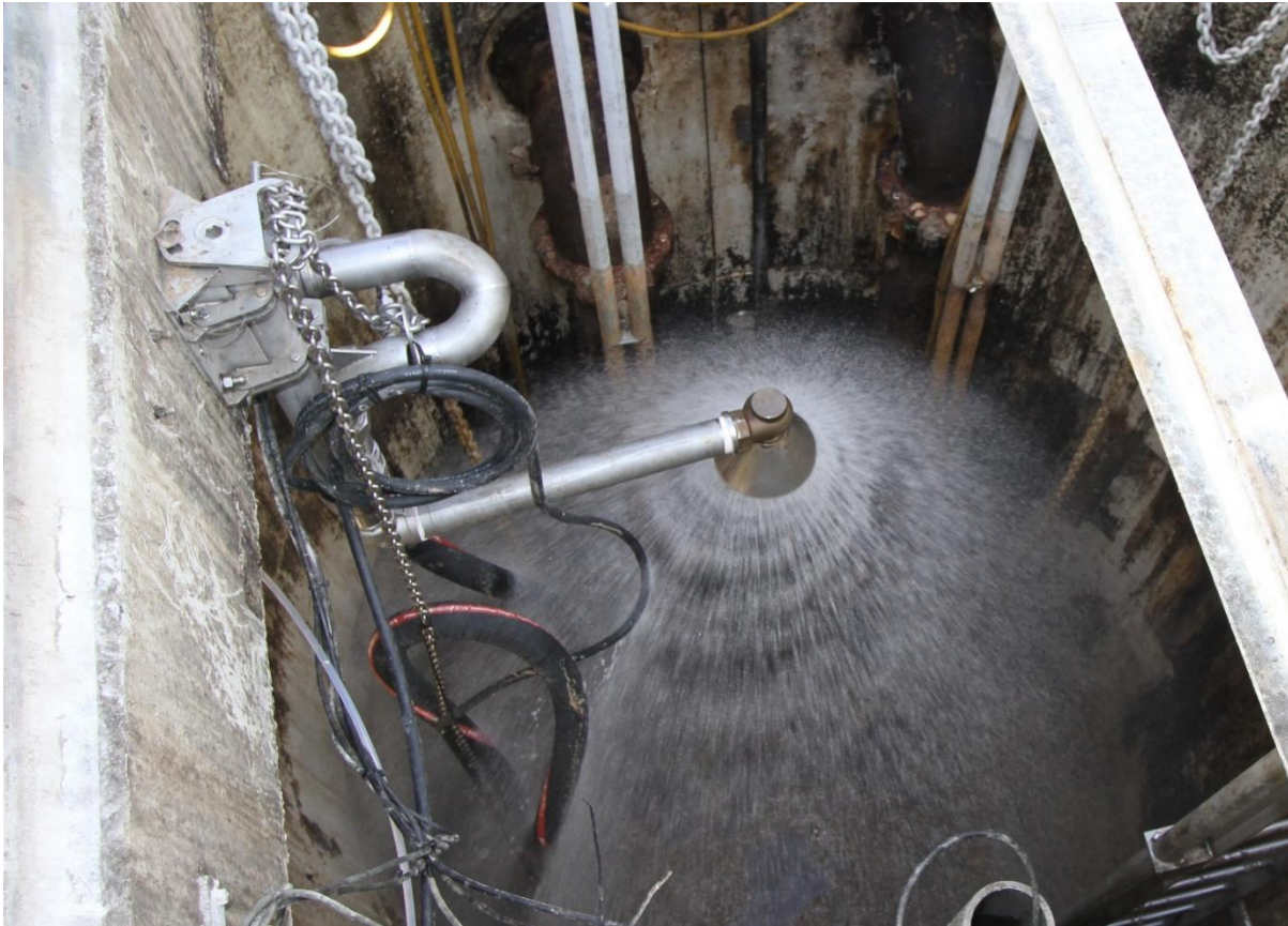
Photograph 10: Example of infuser and spray inside well
