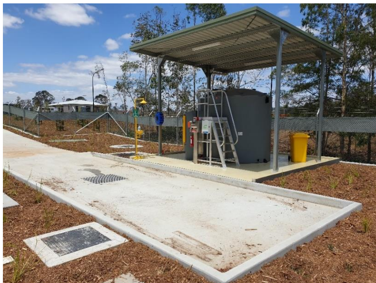
Photograph 5: Example of typical Ferric Chloride dosing unit
