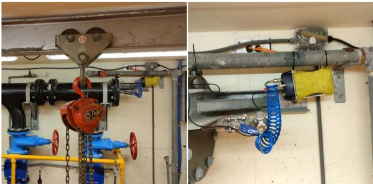
Figure 4: PT Monitor is the yellow unit, installed in a wastewater pumpstation in Seatoun Wellington.
