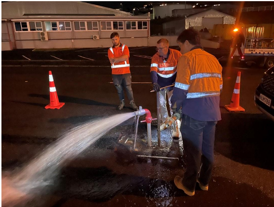
Figure 3: Flushing a hydrant in New Plymouth before connecting p-CAT test kit to the riser
