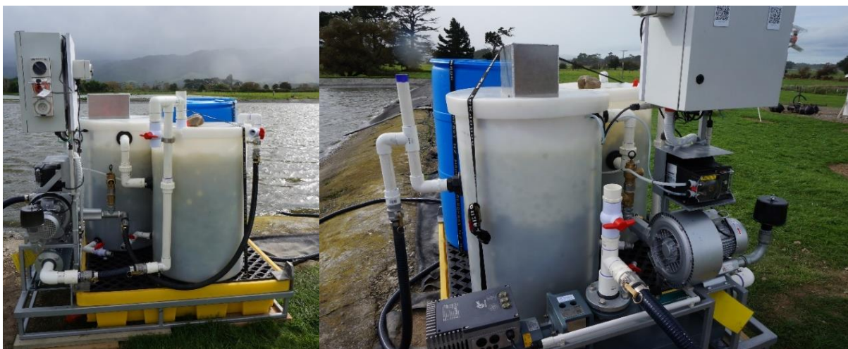
Figure 2: Pilot skid as installed onsite
