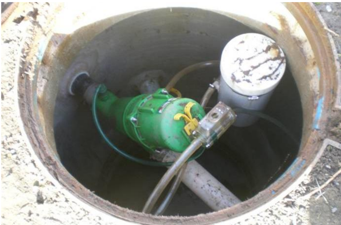
Photograph 3: The vacuum interface valve
