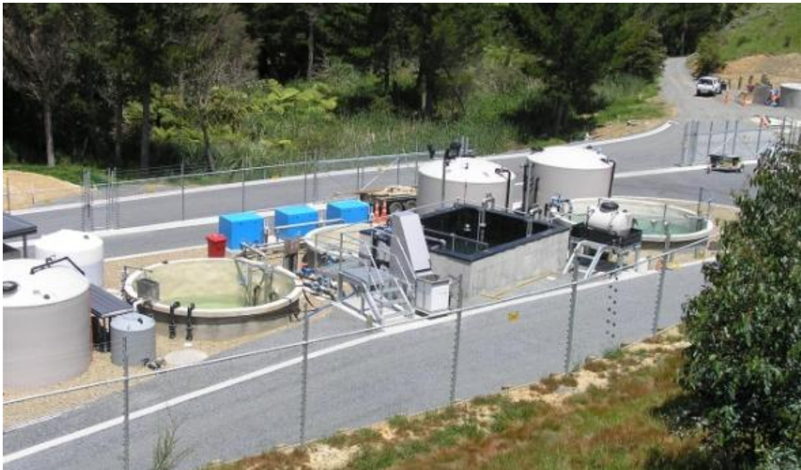
Photograph 8: Secondary Process Treatment area
