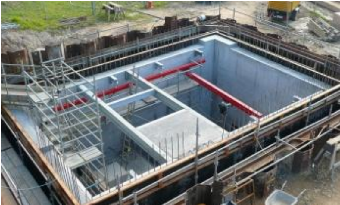
Photograph 6: The vacuum pumping station substructure, 200 m 3 of concrete and 21 tonnes of steel
