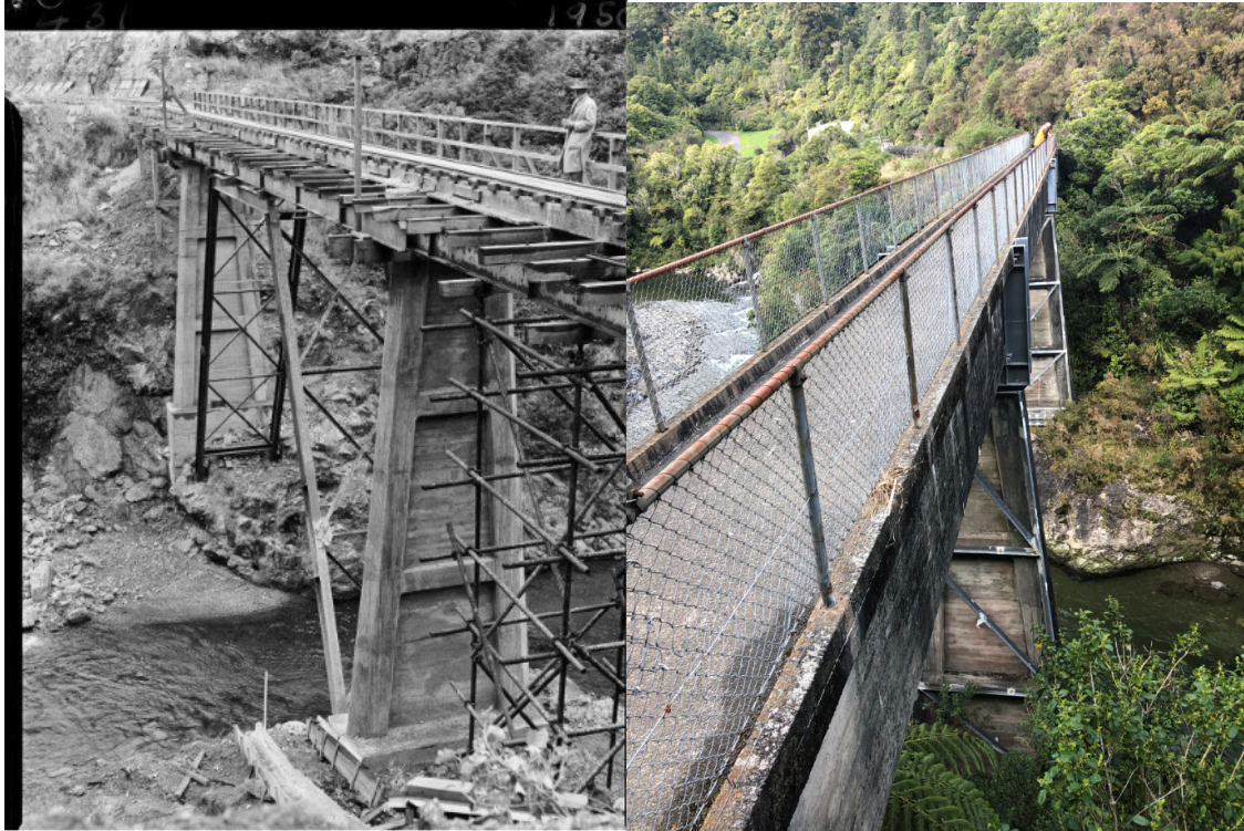
Figure 3: Left photo from the construction of the original bridge, Right photo current condition of the bridge
