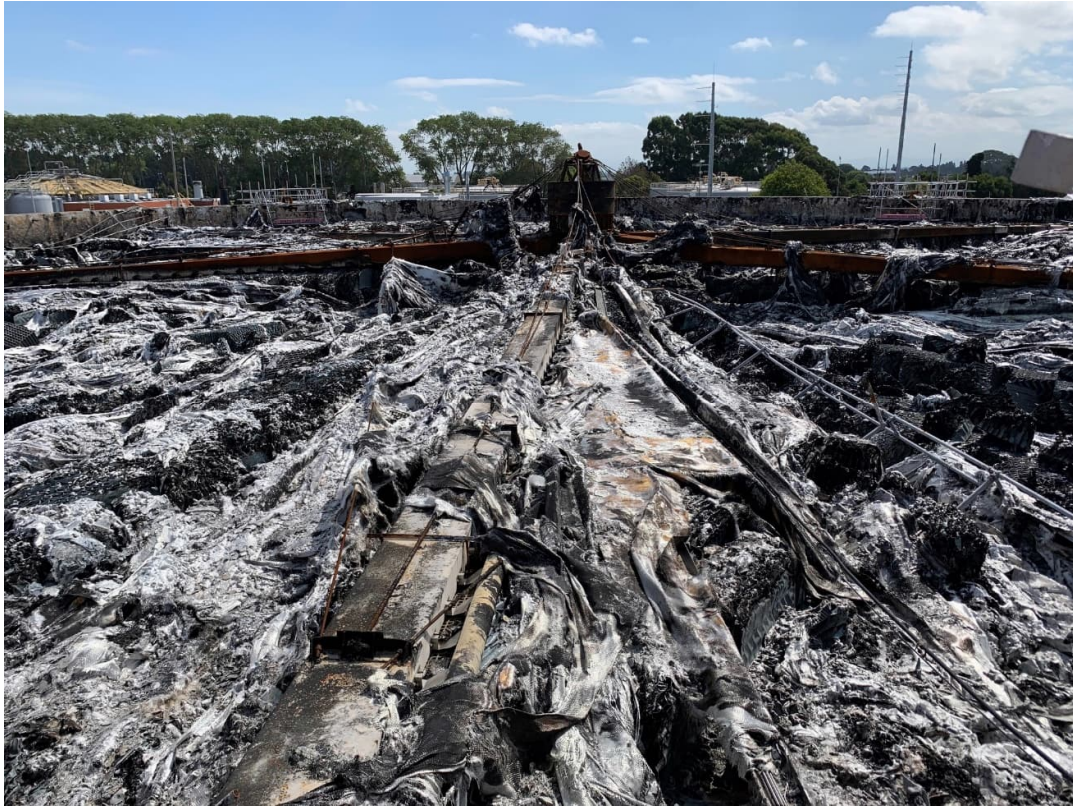
Figure 2: fire damaged trickling filter
