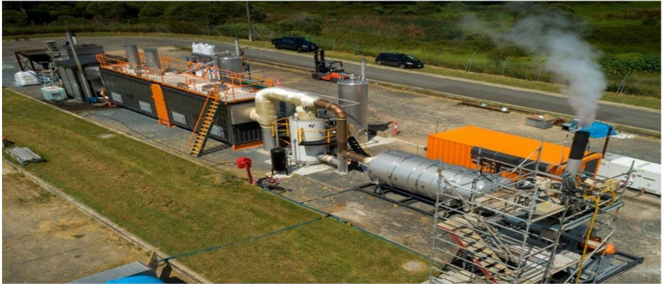
Figure 4-Picture of Loganholme's demonstration biosolid gasification plant
