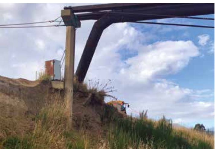
Top: This photo shows the scope of the rock placement required. Above: Erosion of the embankment exposed the pipe bridge foundation.
