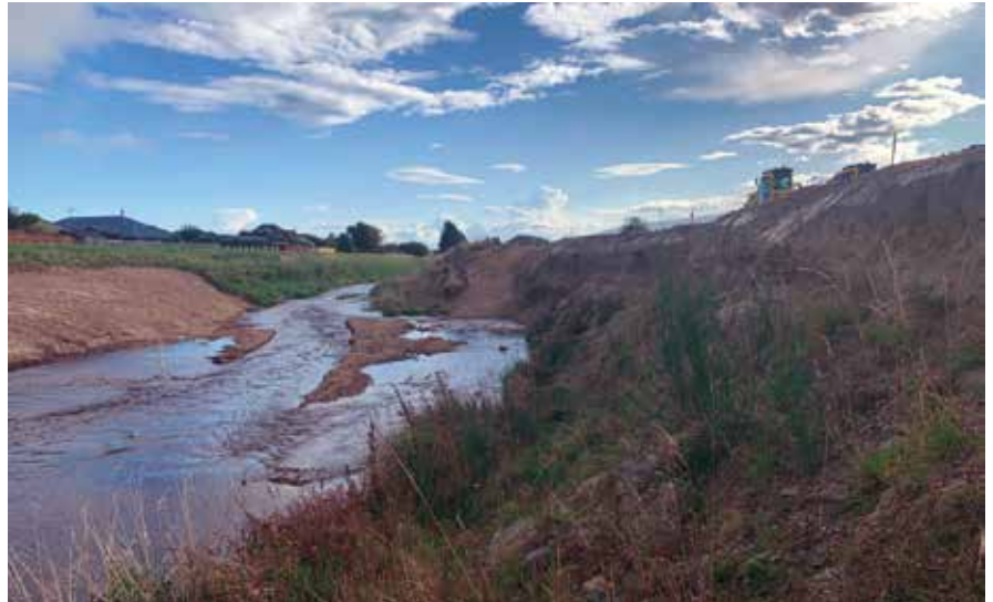
Left: Supervisor Barry Ravenwood, doing a site walkover. Below: A view south showing erosion prior to works. Bottom: The temporary bridge bracing was designed by the internal temporary works team.
