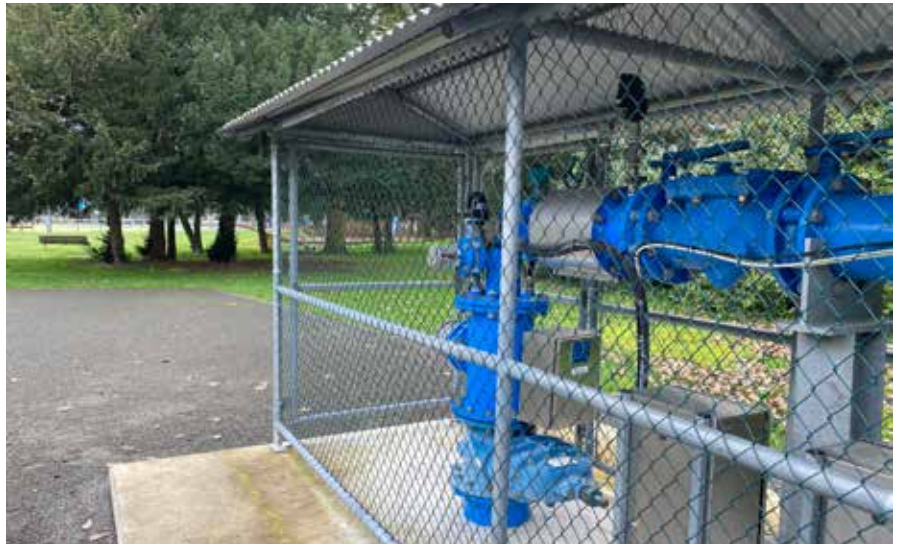
A groundwater monitoring network surrounding a pumping well (such as a public water supply) allows for early contaminant detection and mitigation where possible contaminant source locations are often unknown.
