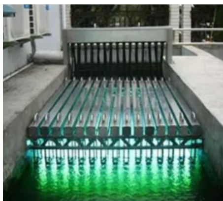
Figure 1: Traditional submerged bulb UV system
