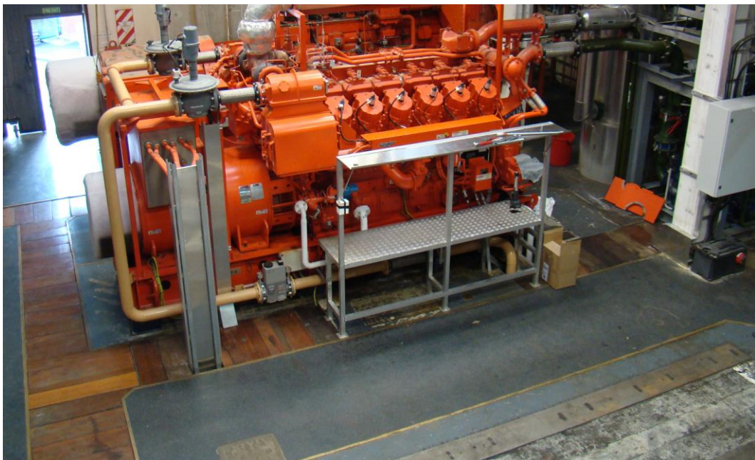
Photograph 2: New 900kW Waukesha
