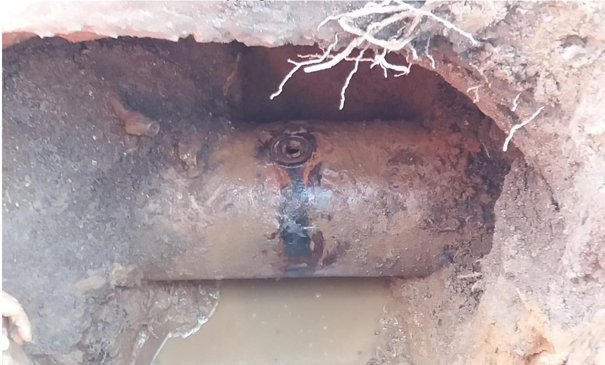
Figure 13: The source of the water leak on Tuhikaramea Road, a 20mm hole where a tapping band had failed
