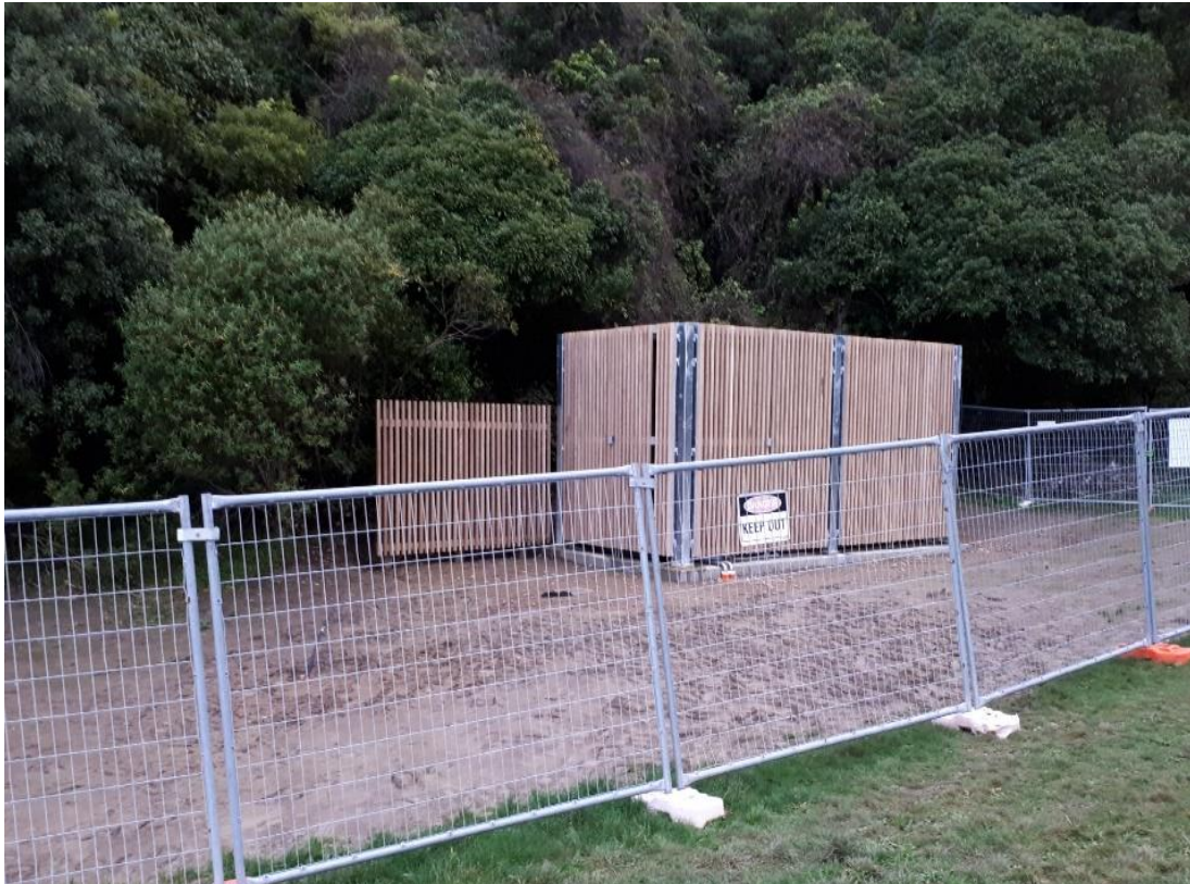
Figure 6: 20ft Containerised Water Treatment plant with facade installed. Wellington Emergency Containers Bore site
