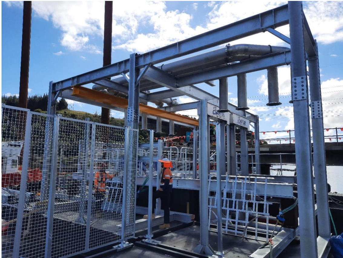
Photograph 8 - Steel gantry frame and monorail
