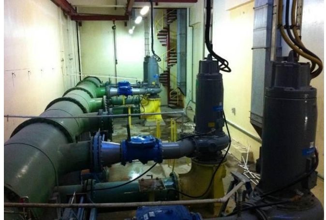
Picture 1 – Beach Road Pumping Station dry well and pumps
