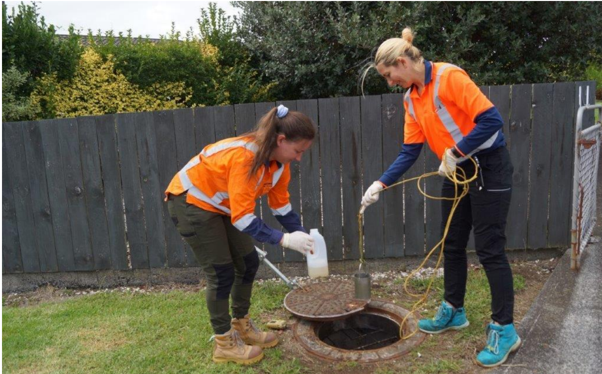
Figure 2 ISCO 3700 composite sampler setup in the drywell at a pumpstation. The inlet hosing threads through the floor and into the wetwell of the pump station. The autosampler is located in the safe location for ease of access.
