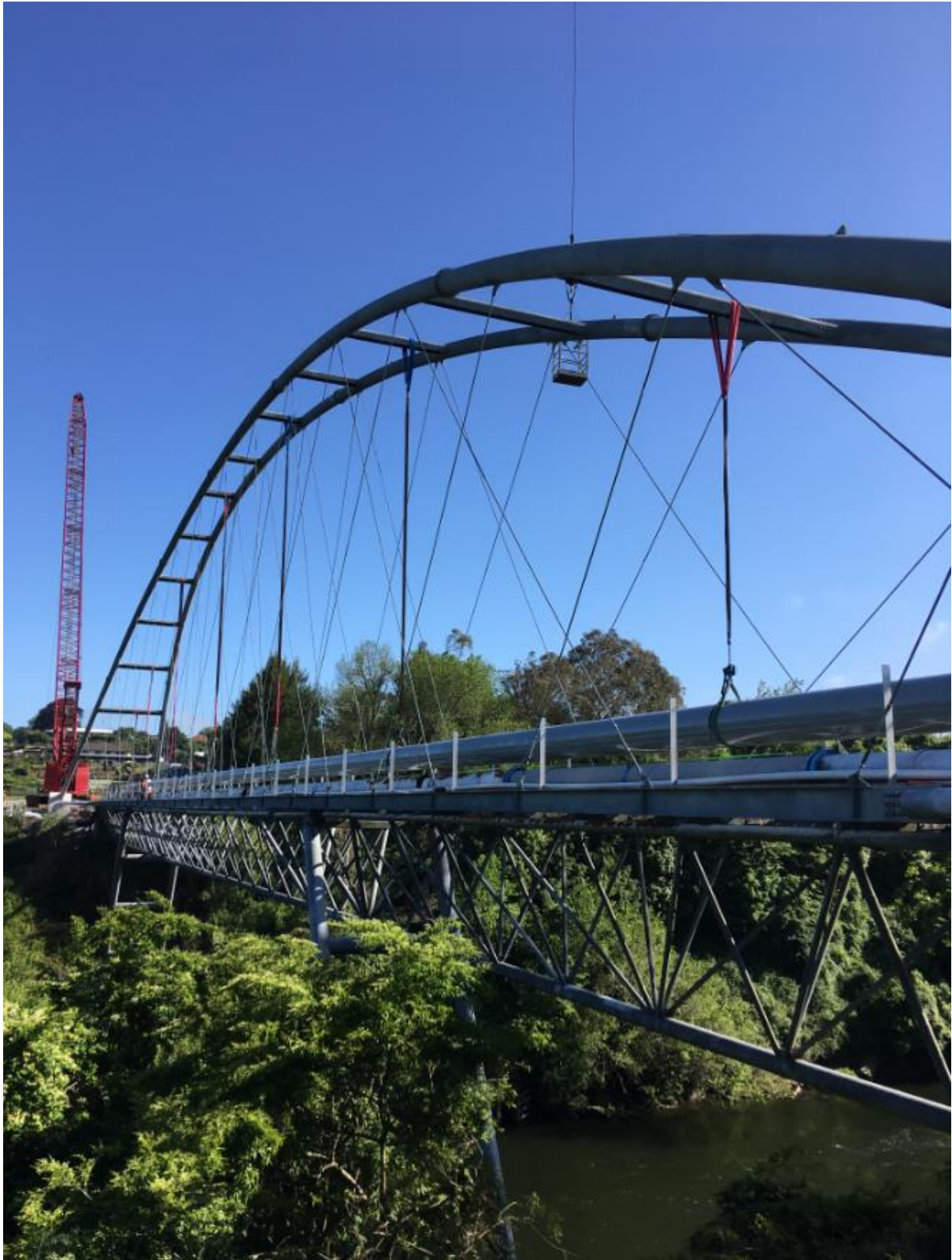
Photo 3: Launching sewer pipework across new bridge structure, original truss bridge below prior to its demolition (November 2018)
