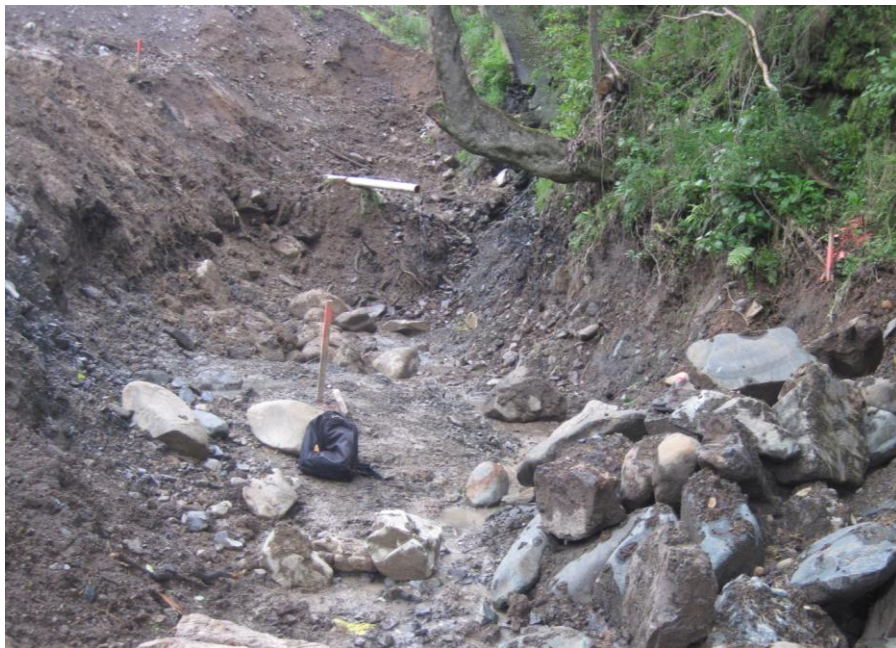
Photograph 8: Leaking cast iron scour pipe with PVC extension (from previous remediation work).
