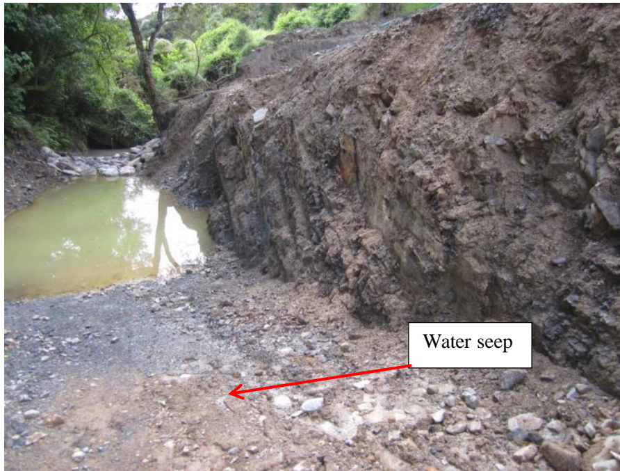
Photograph 7: shows the fractured rock at the stilling basin with water seeping through the rock in the foreground.
