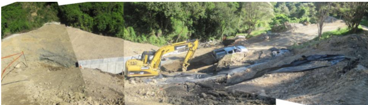
Photograph 10: The site with over half the panels in place. Note the polythene in the foreground protecting the slope from water ingress.
