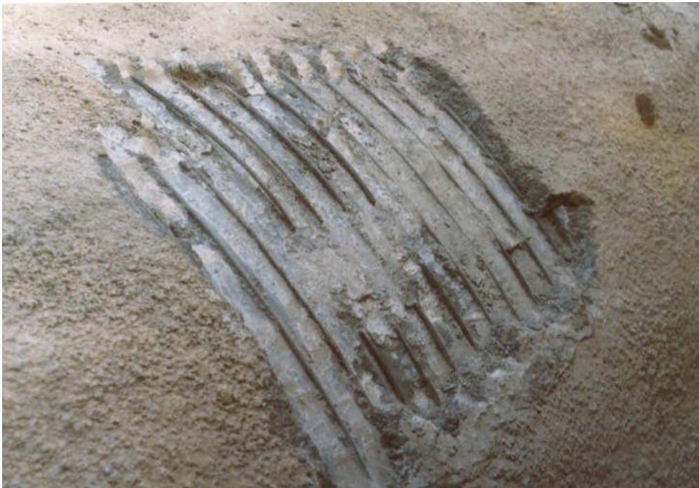
Photograph 1: View of exposed and corroded prestressing wire
