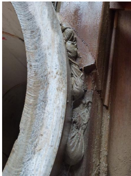
Photograph 7: Annulus Packing – welded plate and sand bag to seal the annulus from ground ingress
