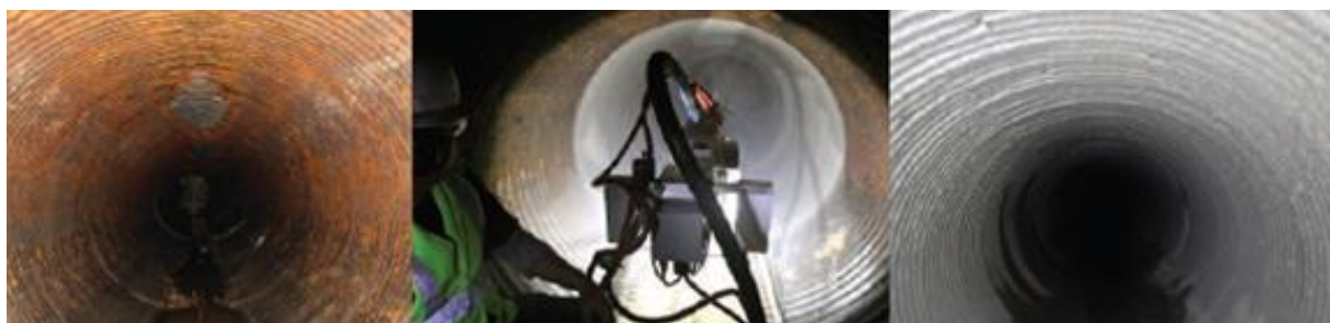
Figure 2: From left to right (a) Leaking storm water culvert (b) Centrifugal application of GeoSpray(c) Completed Repair
