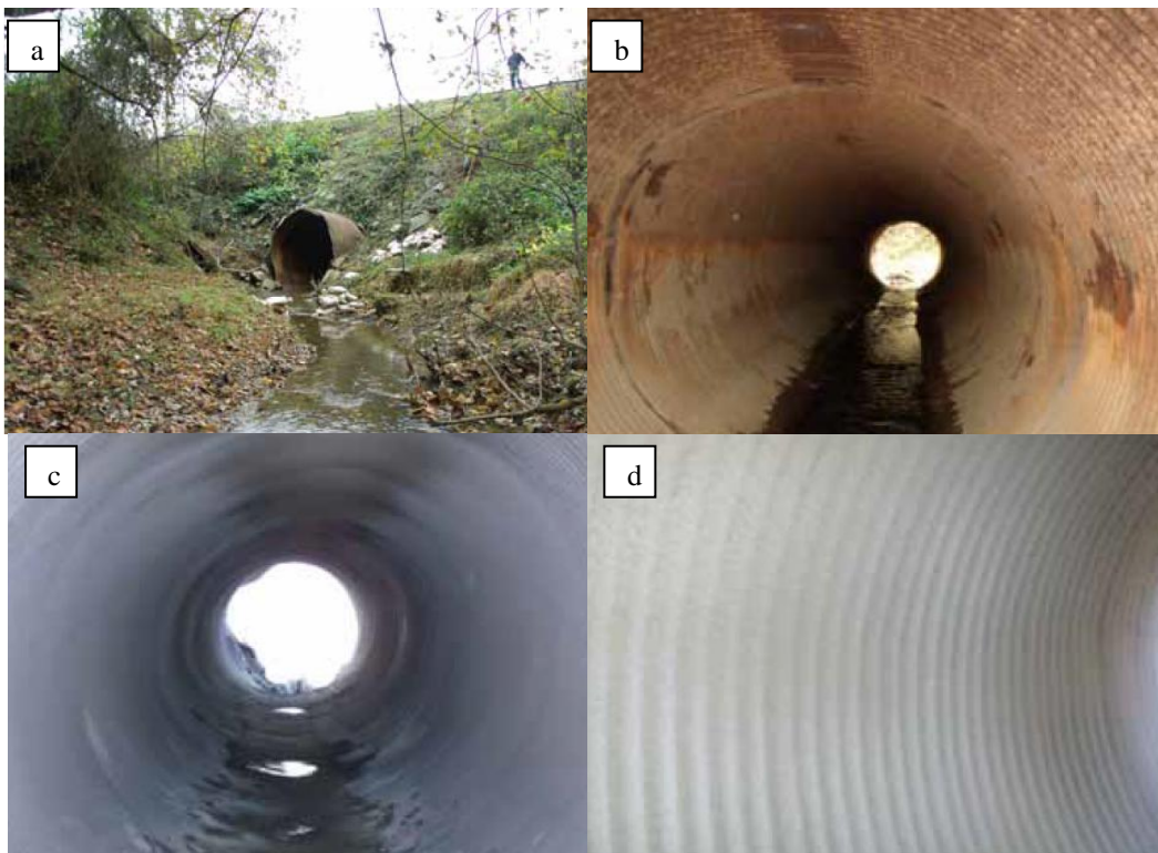
Figure 6: (a) View of Weldon NC Pipe from stream, (b) Pre-rehabilitation condition of pipe, (c) Completed repair, (d) Close up view of CMP wall repair with Geopolymer Lining.
