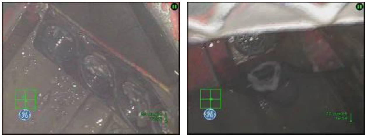
Figure 6. Photo and VDO clips from the inspection of a previous similar project by ICOP
