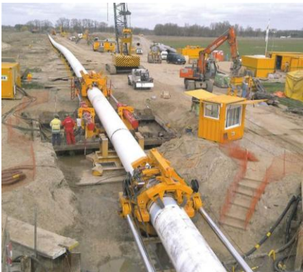
Figure 14: Two HK500PT Pipe Thrusters in line laying a 4,600ft (1,400m) 48" gas pipeline
