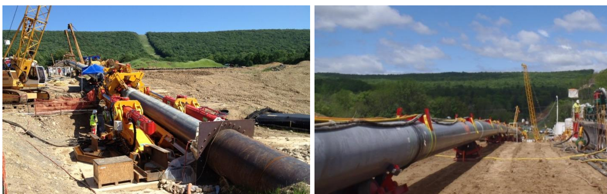
Figure 18 and 19: HK 750PT installed on the launch side in front of the launch pipe – pipe layout section with service lines.
