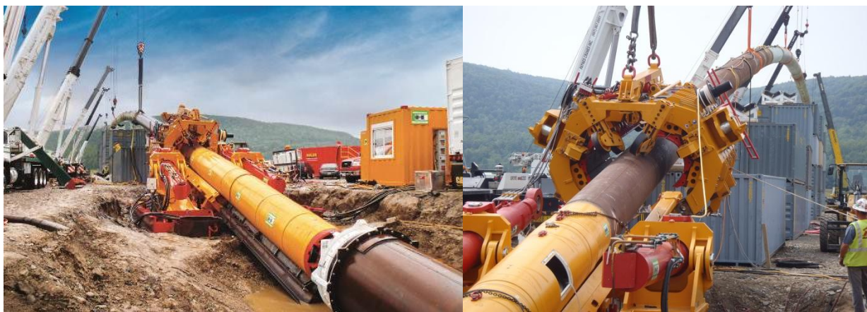
Figure 16 and 17: Pipe Thruster HK750PT anchored on the surface with deployed machine AVN800A and 42” pipeline
