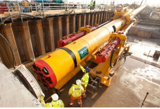
Figure 21: Direct Pipe Equipment set up in the launch pit in front of the launch seal (HK750PT with AVN1200TB) with 56” pipeline.
