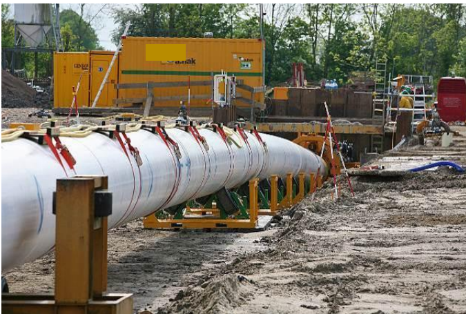
Figure 7: Pipeline (48") laid out on roller supports in the direction of the launch pit.
