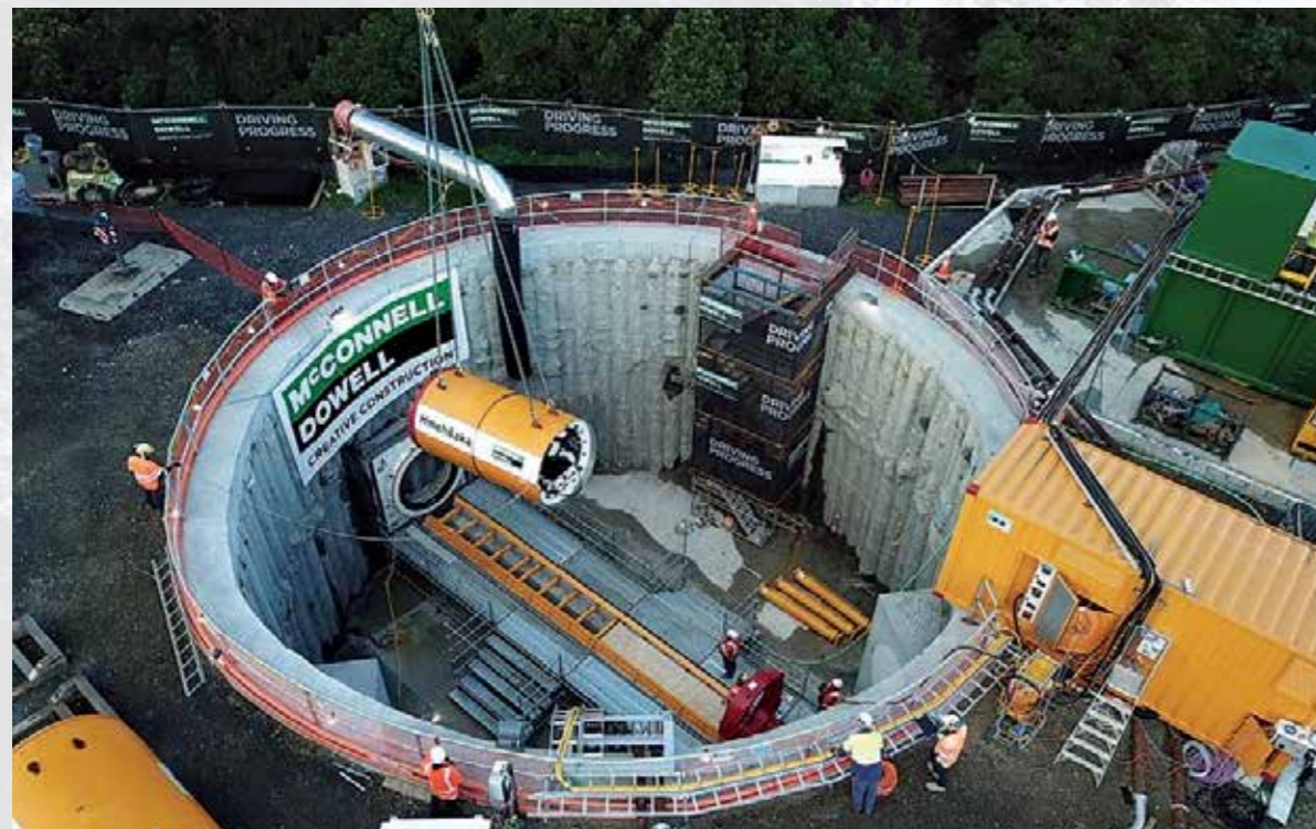
The tunnel boring machine (TBM), Hinehoaka, was tested before she began tunnelling back in early July when it created a new two-kilometres long pipeline for the St Marys Bay Area Water Quality Improvement project in three tunnelling sections or drives.
