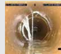
Water infiltration through a pipe defect.
