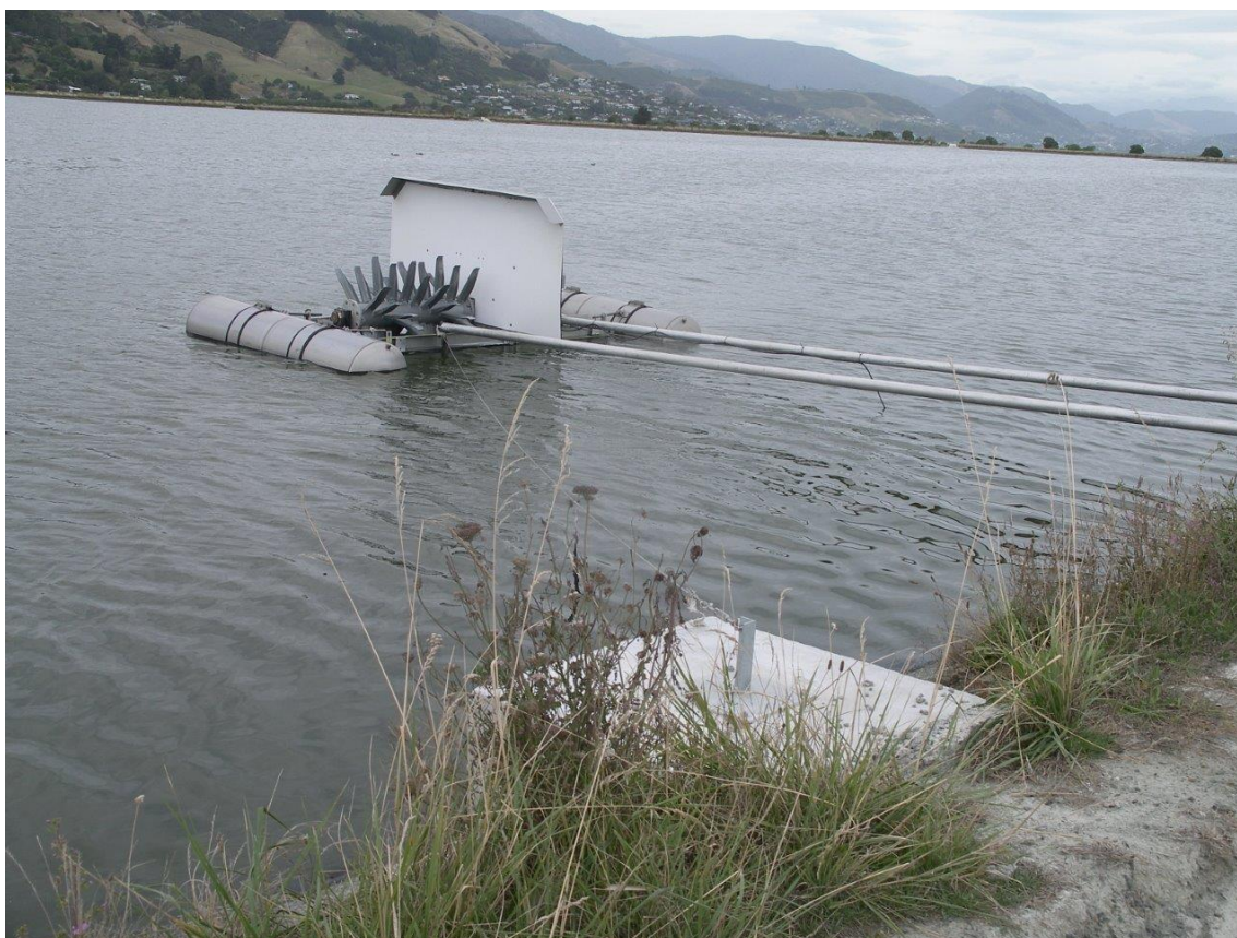
Figure 1 - Brush aerator at Nelson WWTP
