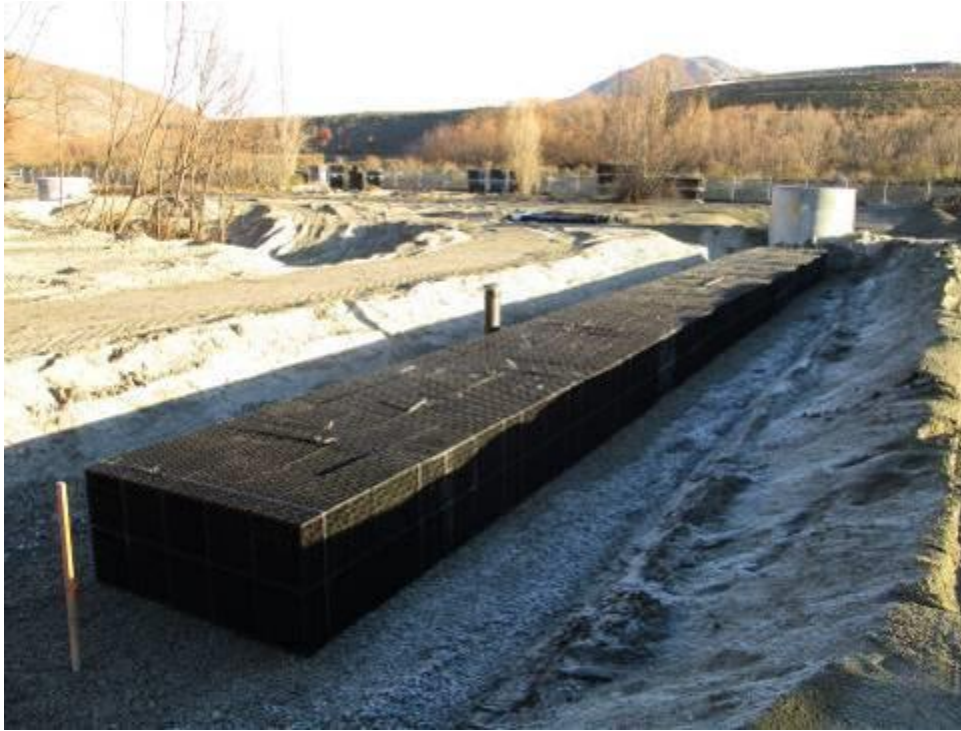
Figure 6: Bed of gravel laid at base of trench, water cells tied together and installed in trench. Monitoring piezometers installed. Manholes installed in centre of each field, above 800 mm dia distribution pipe.
