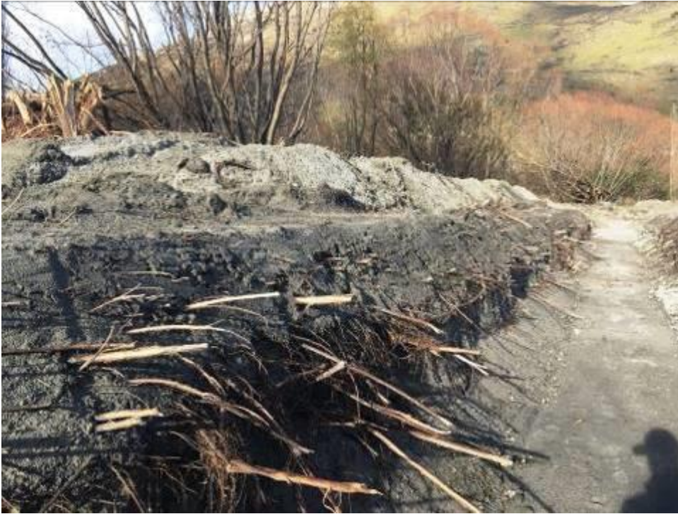
Figure 7: Dense willow root growth in the 800 mm dia pipe trench. The adjacent willow trees were subsequently felled.
