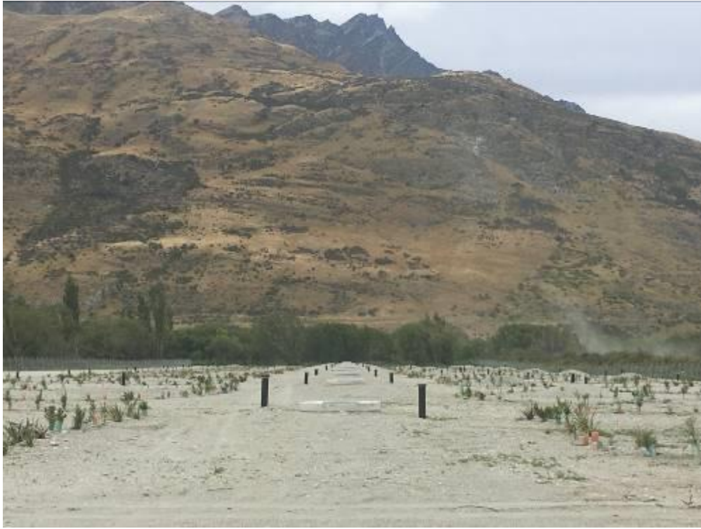
Figure 9: DAD Dispersal field backfilled to finished levels and planted with native species.
