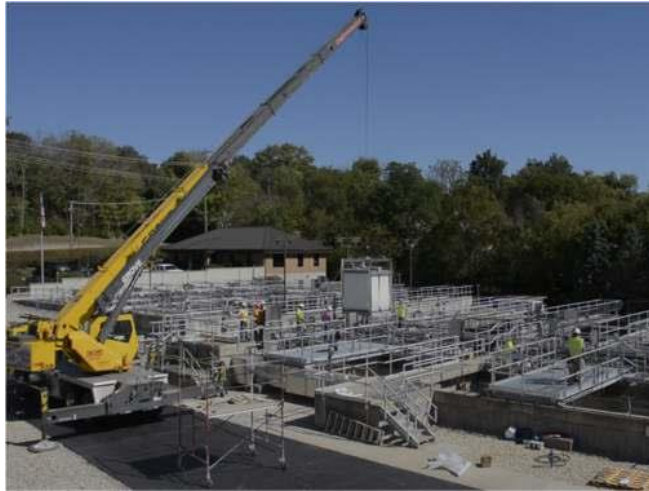
Photograph 1: ZeeLung cassette installation in existing tanks at Yorkville-Bristol Sanitary District
