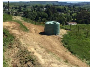
Wastewater Buffer Tank
