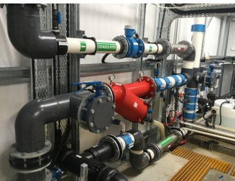
Chemical Injection Points
