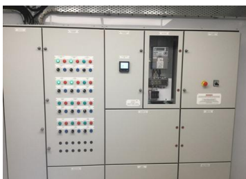
Motor Control Centre
