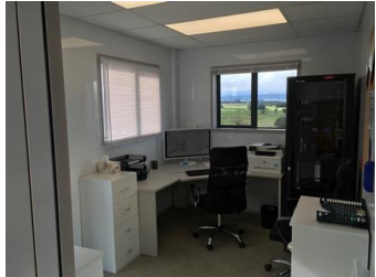
Site Office & SCADA Station
