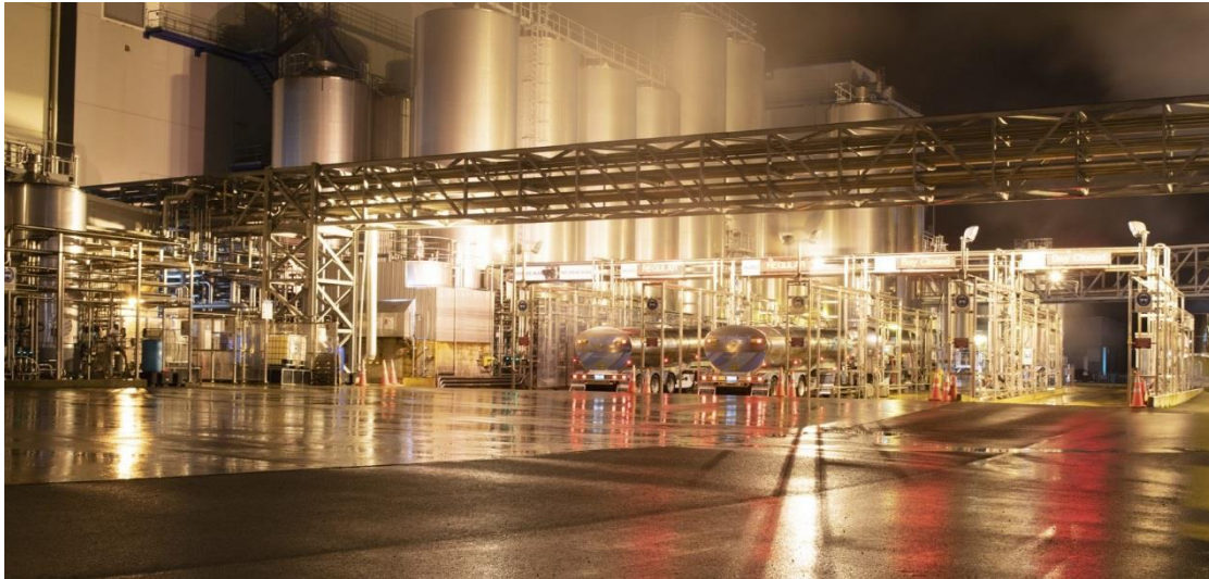
Synlait has switched on New Zealand's First Large Scale Electrode Boiler Photo Source: Synlait 2019
