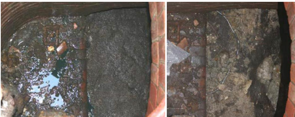
Photograph 3: Results of in network FOG dosing at a secondary manhole.
