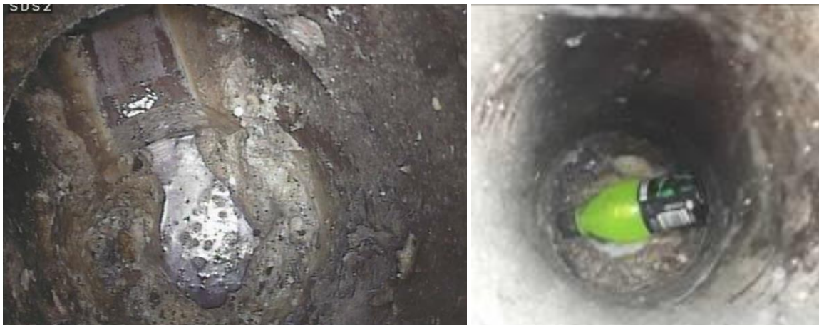
Photograph 6: Examples of Buchan Trap blockages
