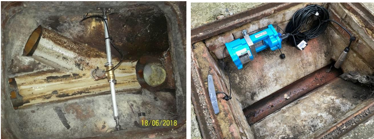
Photograph 4: Property Level alarm installation examples
