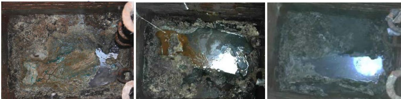
Photograph 2: Results of in network FOG dosing at a manhole over 3 months.
