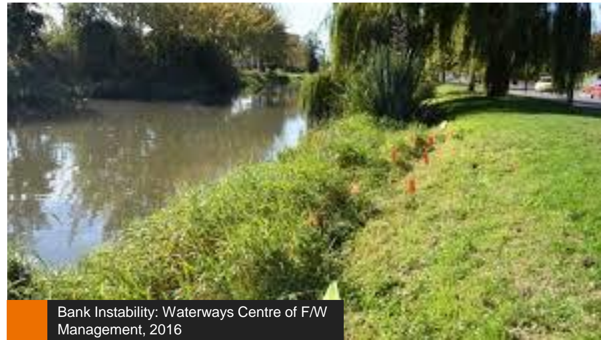
Bank instability: EOS Ecology, 2011
