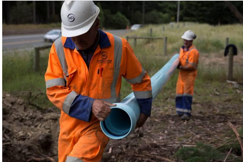
Photograph 4: Site handling a 6.5 m length of DN200 Series 2 PVC-O (Image courtesy – Iplex Pipelines NZ Limited)
