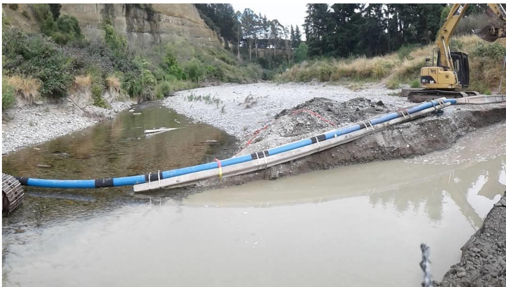
Photograph 7: Waianakarua River Crossing utilising concrete poles for anchorage. (Image courtesy – Waitaki District Council & Whitestone Contracting)
