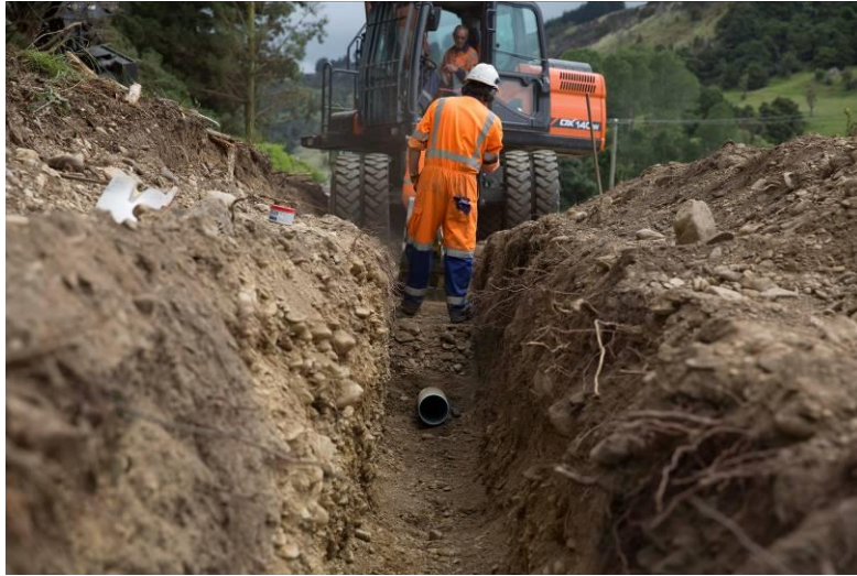
Photograph 6: Compaction of embedment zone above pipe (Image courtesy – Iplex Pipelines NZ Limited)
