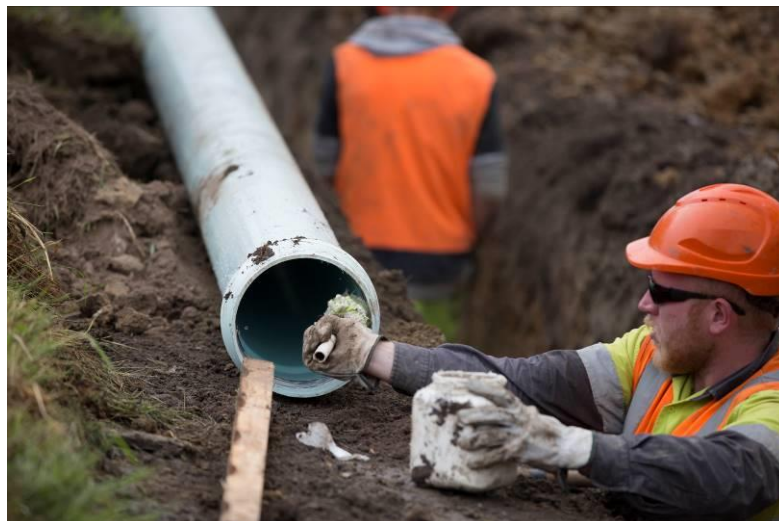
Photograph 5: Application of bactericidal pipe jointing lubricant to the locked-in-place seal ring (Image courtesy – Iplex Pipelines NZ Limited)
