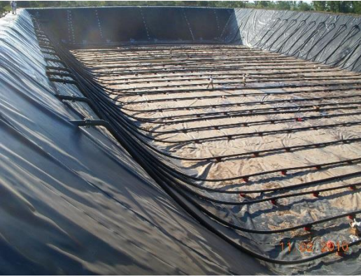
Photograph 1: Photo of feed and sludge removal pipe on an engineered lagoon digestion system.
