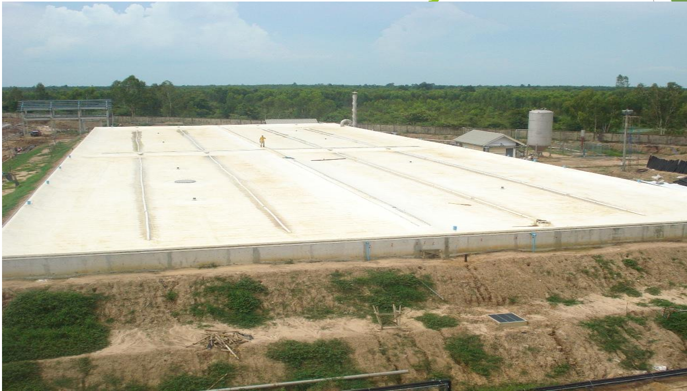
Top view of the low-rate anaerobic treatment system
