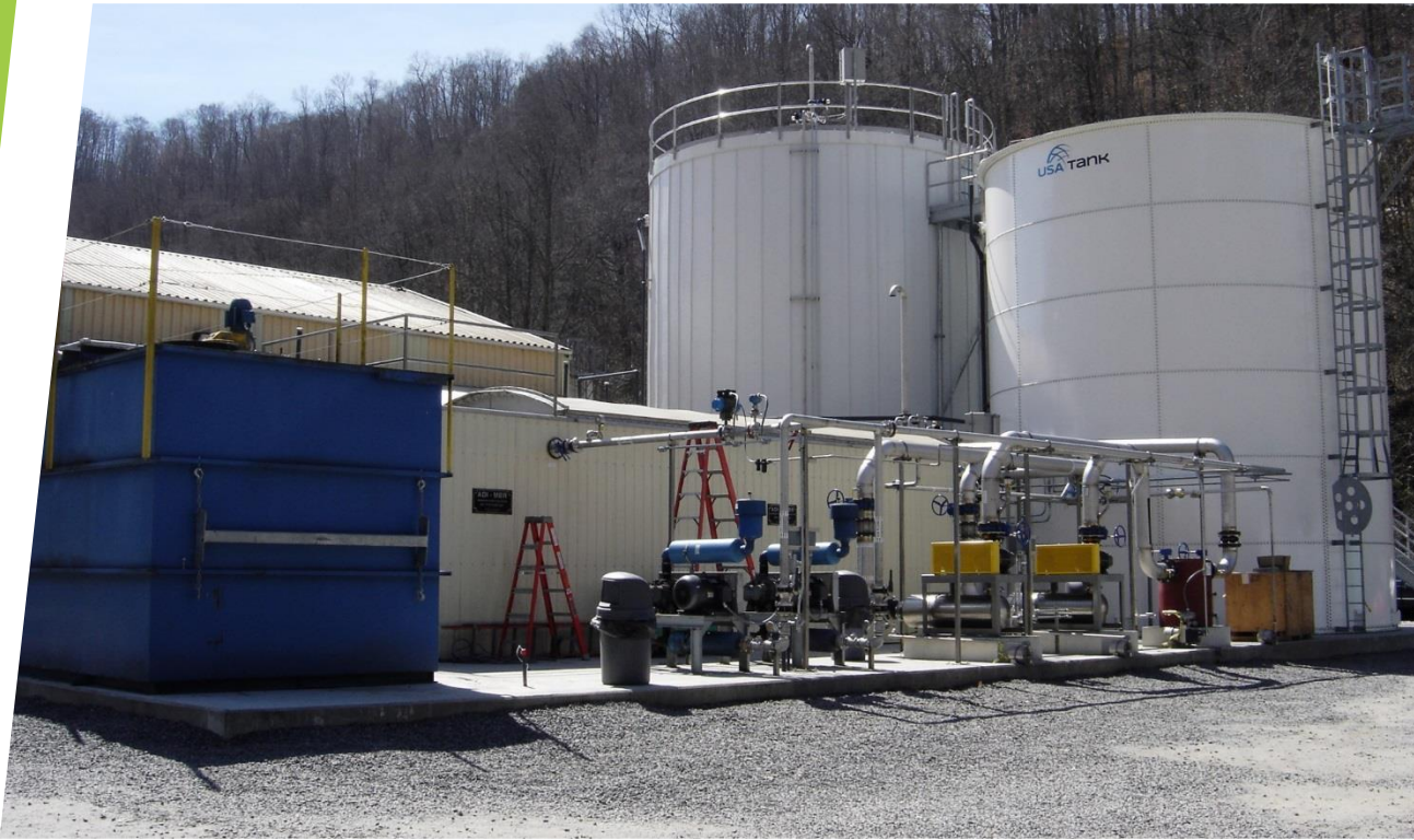
Pop tart plant - Kentucky AnMBR / MBR Bio-Reactor
