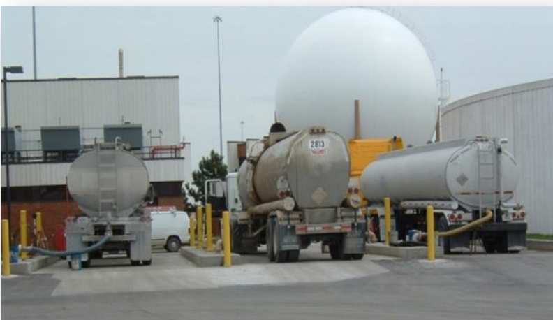
Figure 20 – Truck Loading Facility for Receiving Organic Waste
