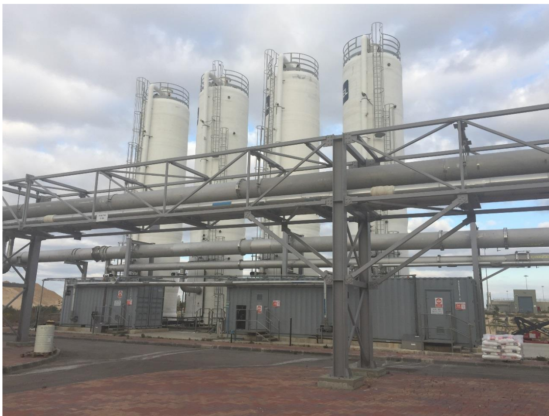
Figure 12 – Biological Hydrogen Sulfide Removal System
