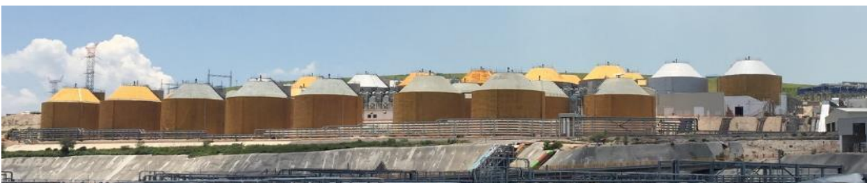
Figure 1 – Thirty Mesophilic Anaerobic Digesters at Atotonilco
