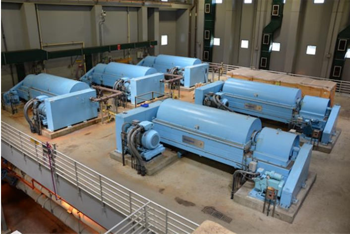
Figure 6 - Picture of five thickening centrifuges to be replaced
