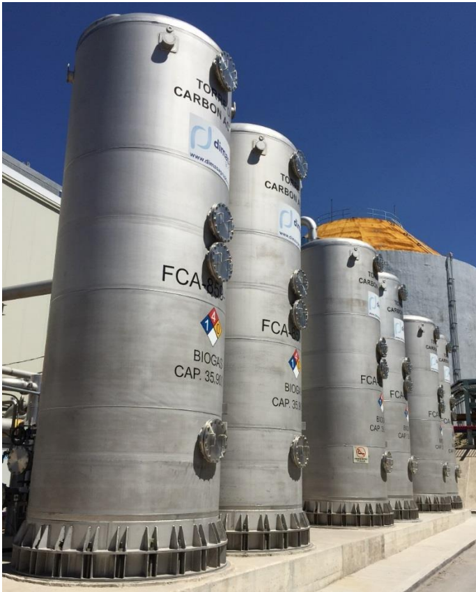
Figure 4 – Activated Carbon Vessels for Gas Treatment at Atotonilco
