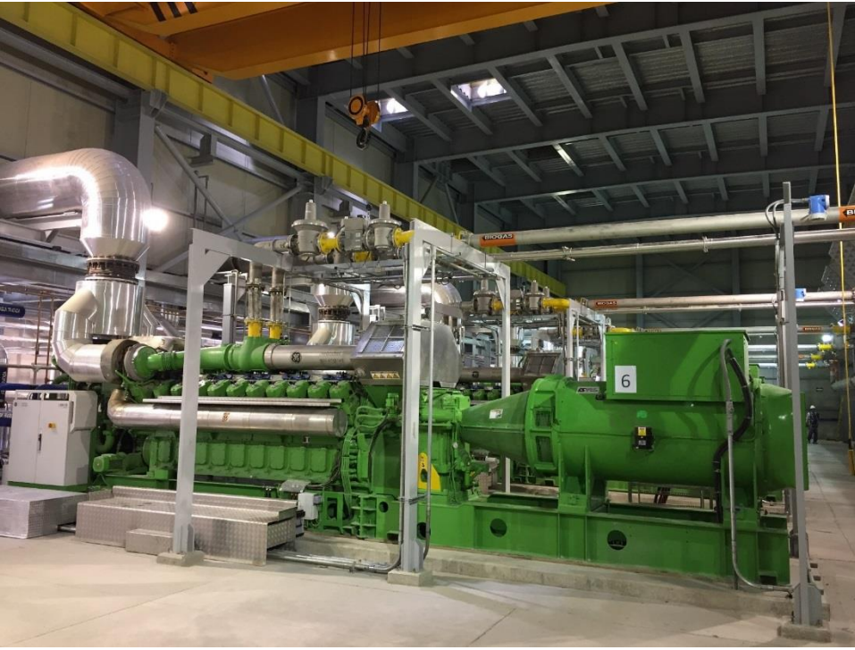
Figure 2 – One of Twelve CHP units at Atotonilco
