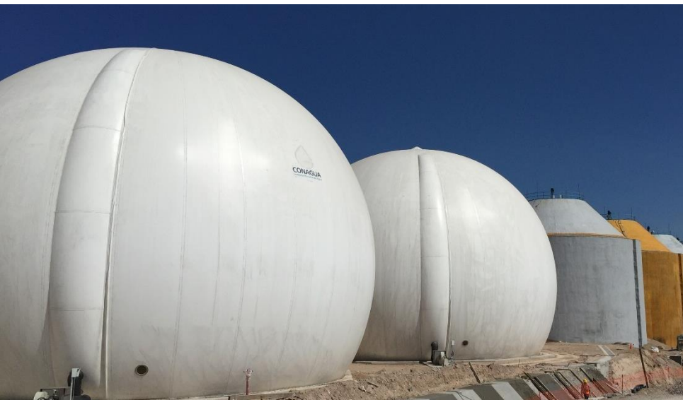
Figure 3 – Membrane Gas Holders at Atotonilco
