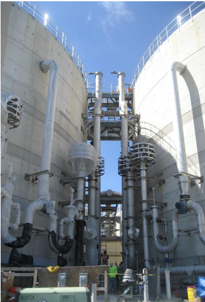
Figure 18 – Standpipes and Emergency Overflow Piping
