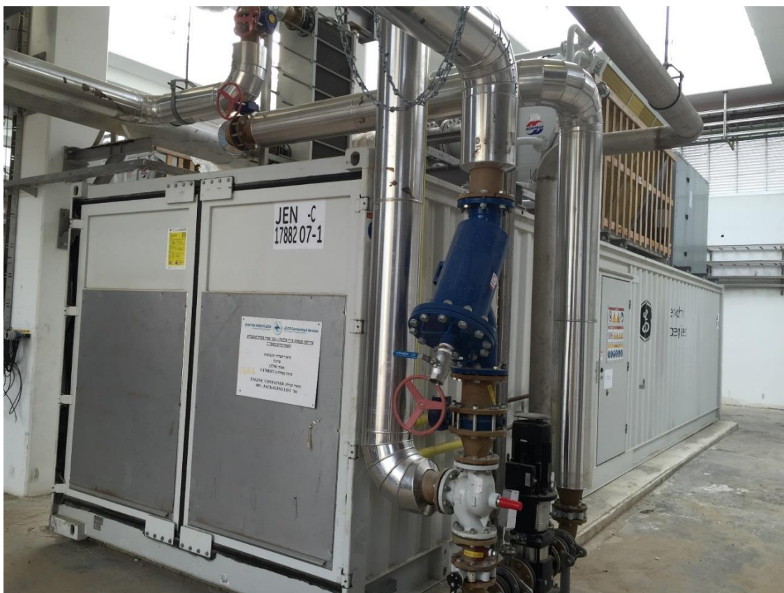
Figure 11 – One of the 1.4 MW Cogeneration Units
