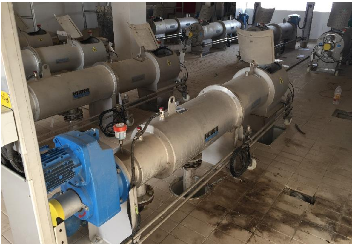
Figure 10 – Shafdan Primary and Secondary Sludge Screens
