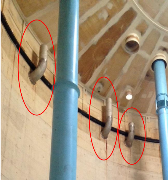
Figure 17 – Three Sludge Withdrawal Pipes in the Digesters
