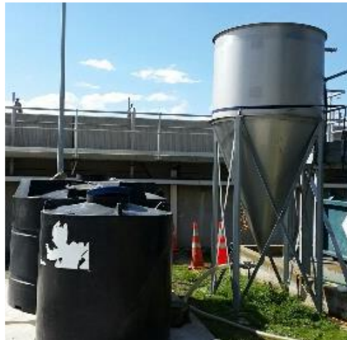
Photograph 1: Pilot Trial Sludge Thickening Tanks
