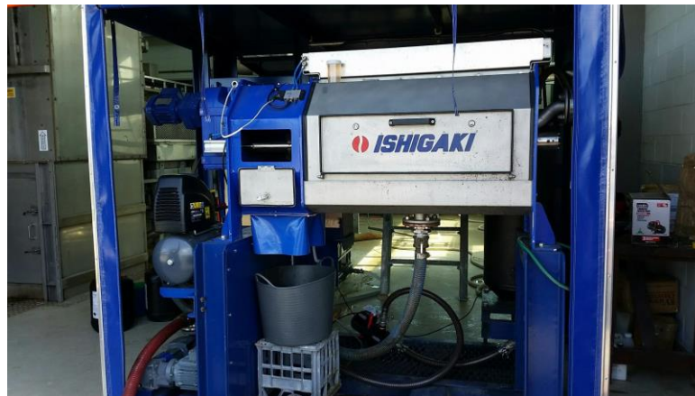
Photograph 2: Screw Press Pilot Plant Unit
