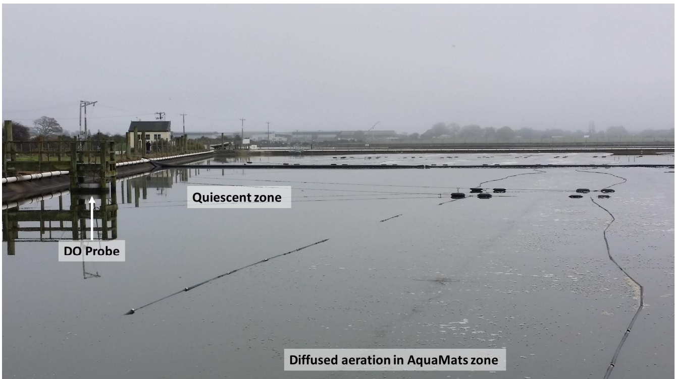
Figure 11: Location of DO Probe in Quiescent Zone at Matamata WwTP
