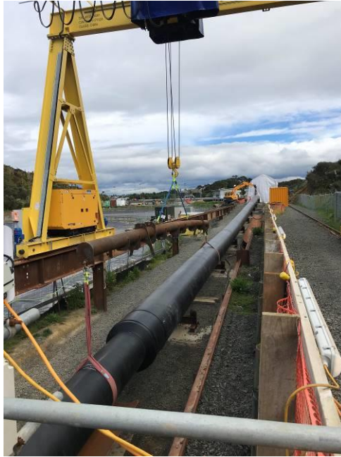
Figure 20: Butt fusion welder in white tent and gantry helping liner down to the tunnel
