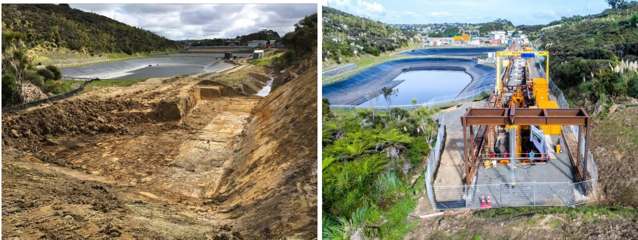
Figure 6: On the left a photo of the site at the early stages of earthworks, on the right a photo at full mobilization.
