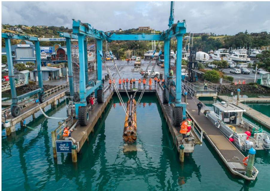
Figure 13: MTBM hoisted into the air by the Gulf Harbor Marina Straddle lift
