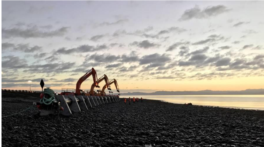
Figure 16: Three 30t excavators working in tandem at low tide to launch the 1 st String
