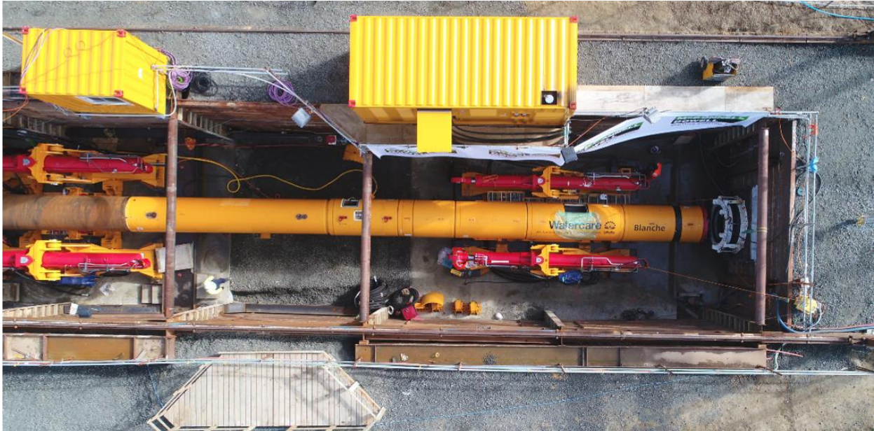
Figure 3: Overhead view of the Direct Pipe® Machine before launch – 500t thruster at the front and 750t thruster at the rear.
