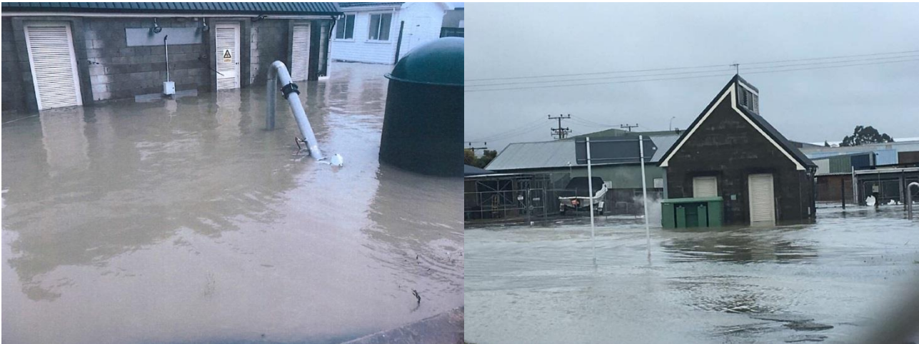
Photograph 1 & 2: Beach Road Pump Station inundated by storm surge
