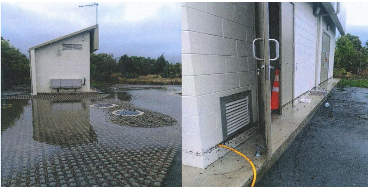
Photograph 3 & 4: Songer Street Pump Station (with water mark)
