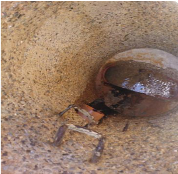
Figure 14: Manhole with exposed aggregate from H 2 S attack
