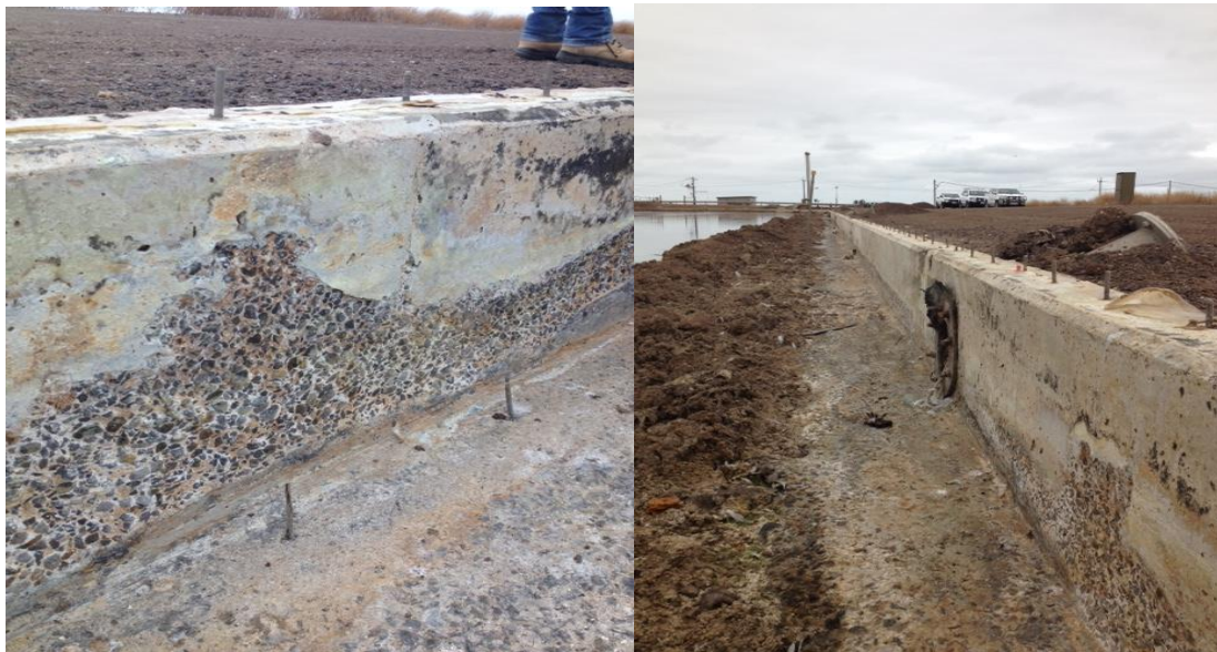
Figures 3 & 4: Depicts degradation to cement paste from H 2 S attack
