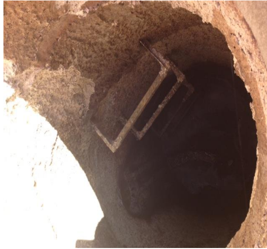
Figure 5: Manhole with significant deterioration from H 2 S attack
