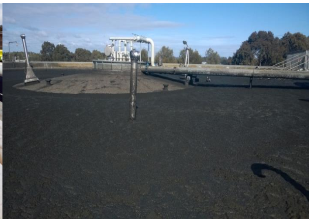
Figure 13: Digester back in service
