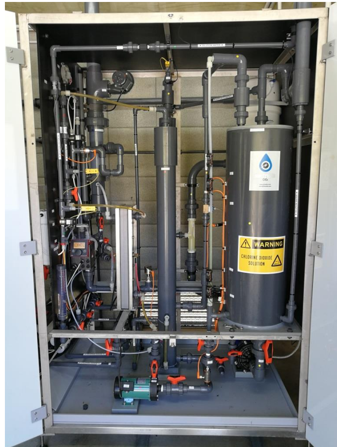
Photograph 1: Patea Chlorine Dioxide Generator
