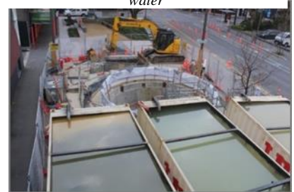
Figure 25: Storage of contaminated ground water
