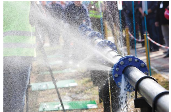
Figure 5: Burst pipe – so what?
