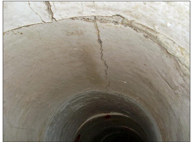
Fig 2: Cracks in the top of a reinforced concrete culvert
