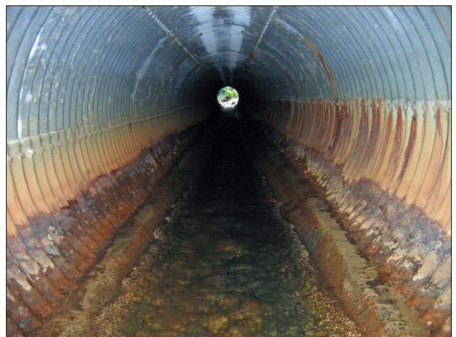
Figure 5: Concreting the invert of a culvert can extend its life, but ultimately moves corrosion and abrasion problems further up the wall.
