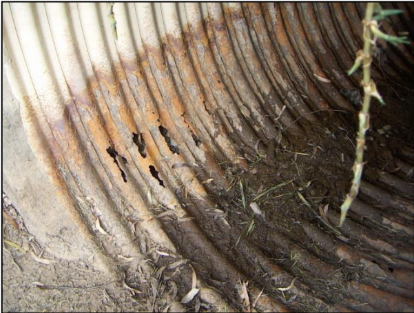
Fig 1: Perforations in the rusted invert of a corrugated metal culvert
