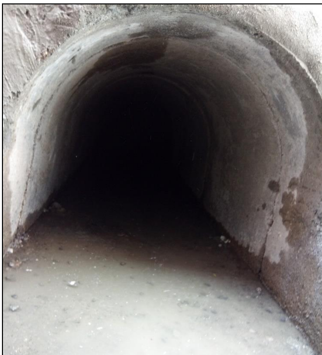
Figure 10: Non-circular culvert subject to deterioration and heavy siltation
