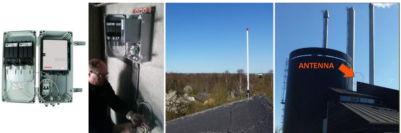
Figure 14 AMR concentrator and antenna
