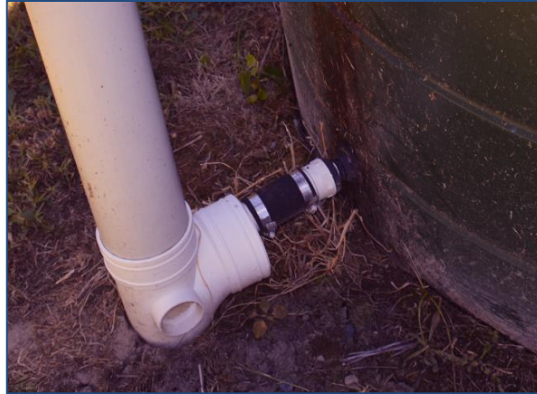
Photographs 21: Difficult to maintain stormwater tank
