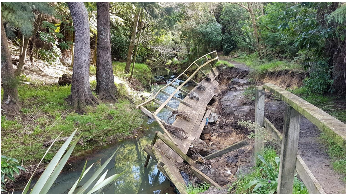
Figure 1: Collapsed retaining wall and walkway caused by streambank erosion occurring at Oakley Creek
